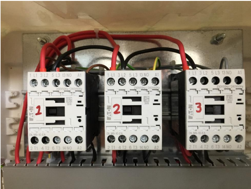
Figure 9: Temperature control unit contactors.
