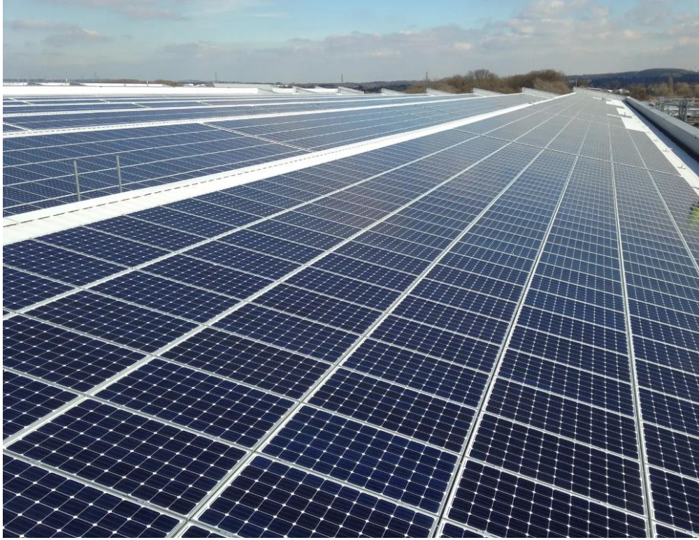
Figure 95. Array of Solar Panels
