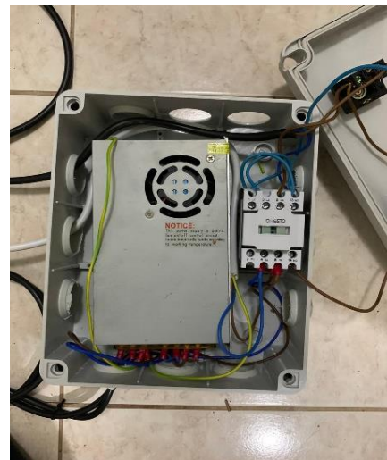
Figure 3.1-13 Control Box interior
